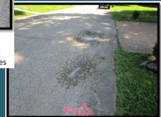
Garibaldi Place: Alligator Cracking w/ Potholes
