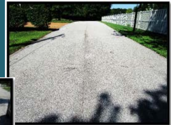
Donoho Place: Longitudinal & Transverse Cracking
